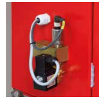
Pressure recorder transducer and run test solenoid valve
